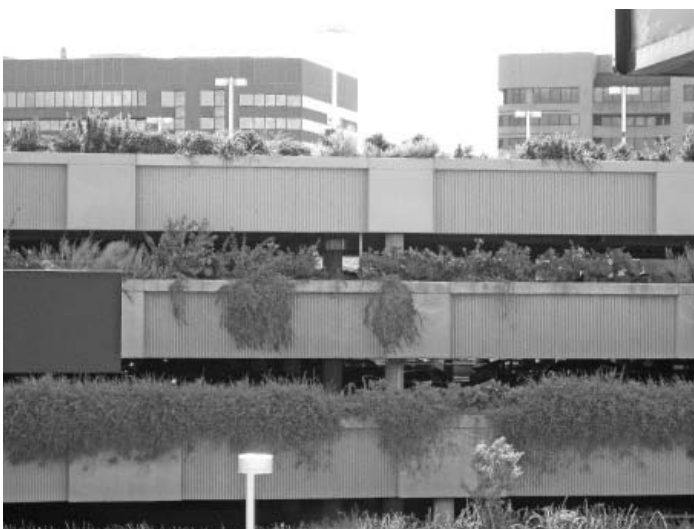
Photo 3.8: Infiltration through greening of car park in Washington, DC. Source: J Lamond
